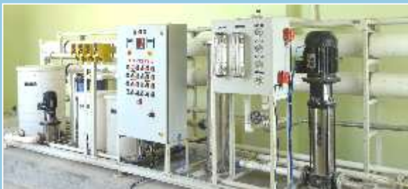
RO Plant at CTS Siruseri
