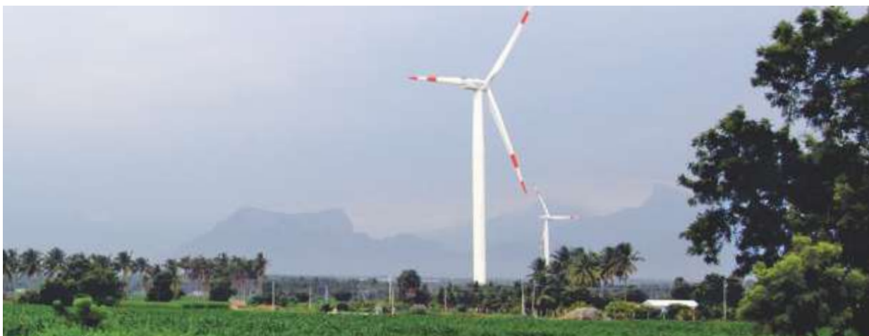
Wind Electric Generator installed by L&T near Coimbatore
