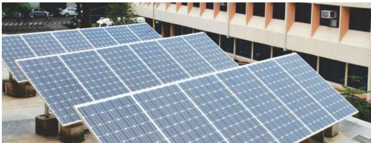
Solar PV panels installed at Powai campus
