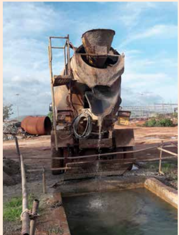
Waste Water Collection Tank
