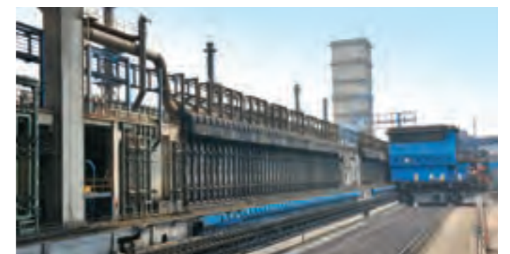
Coke oven battery executed by L&T for one of India's major steel plants.
