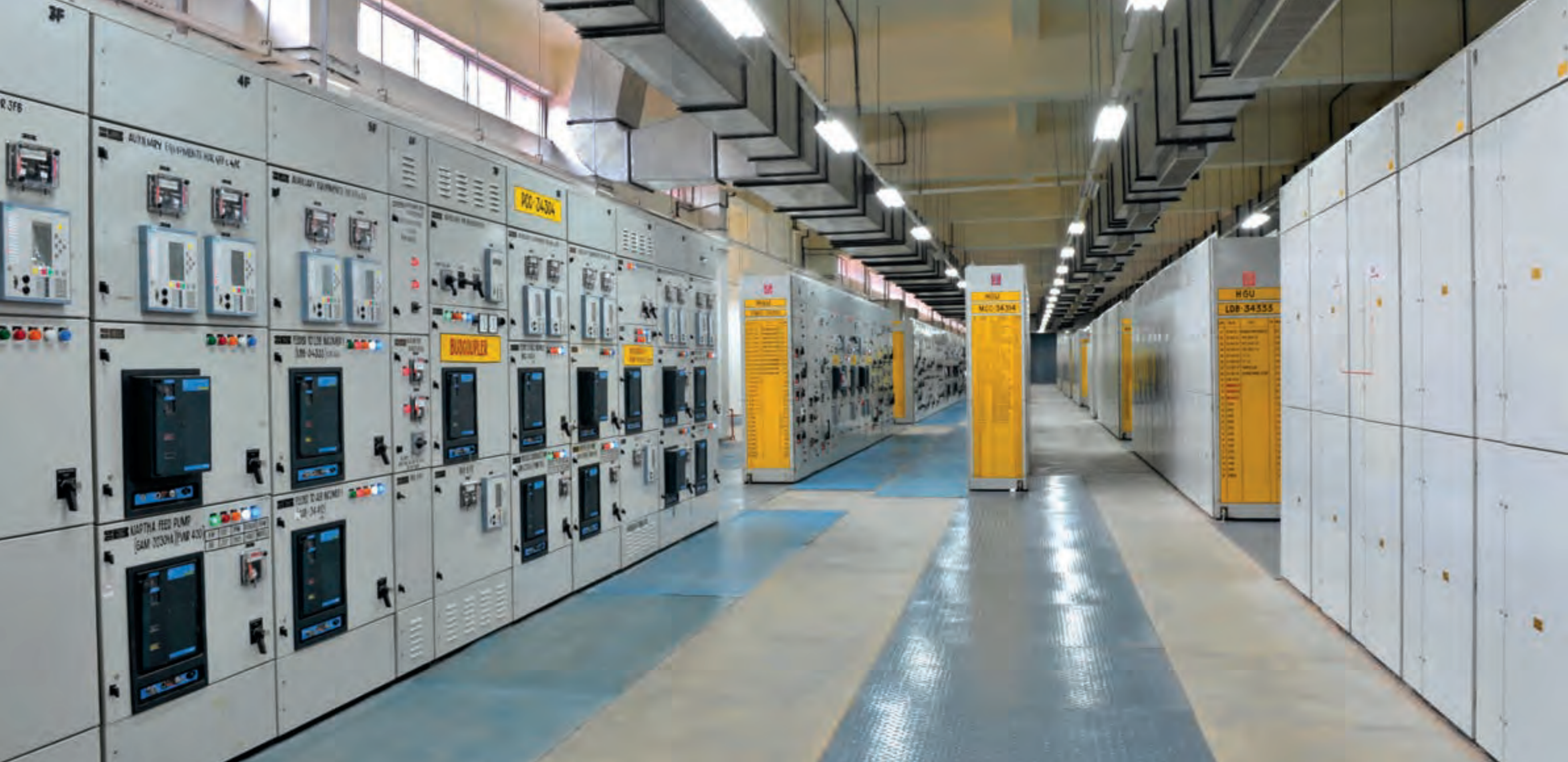
Switchboard installation at a power plant. L&T provides power distribution and control solutions – including LV and MV switchboards – across the value chain, from point of generation to end-user.
