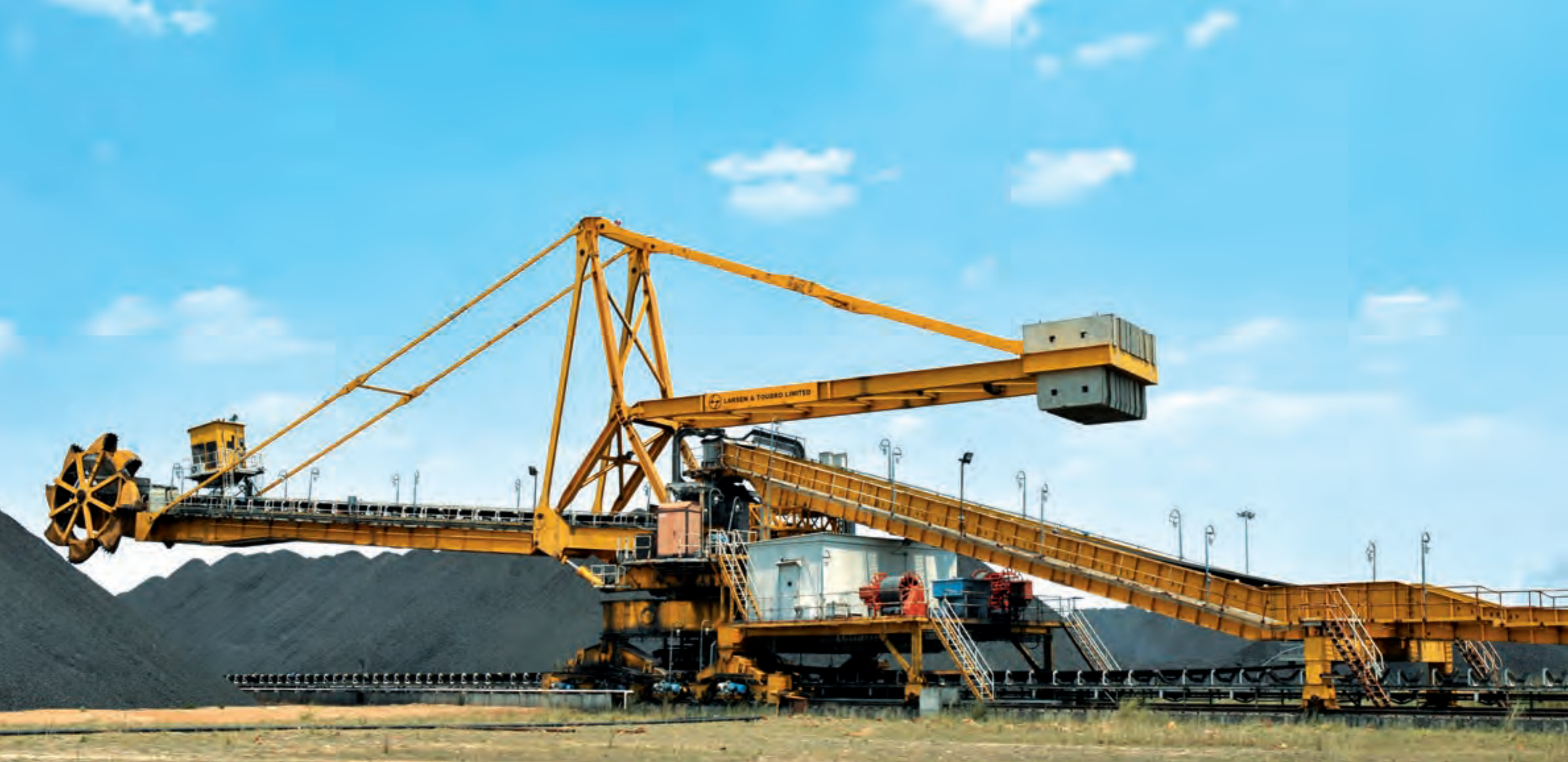
Coal-handling plant executed by L&T at Koderma in Jharkhand. L&T is a single-point solutions provider for a comprehensive range of material-handling systems.
