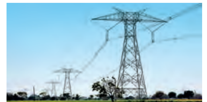
800 kV transmission lines between Nidhura and Agra.
