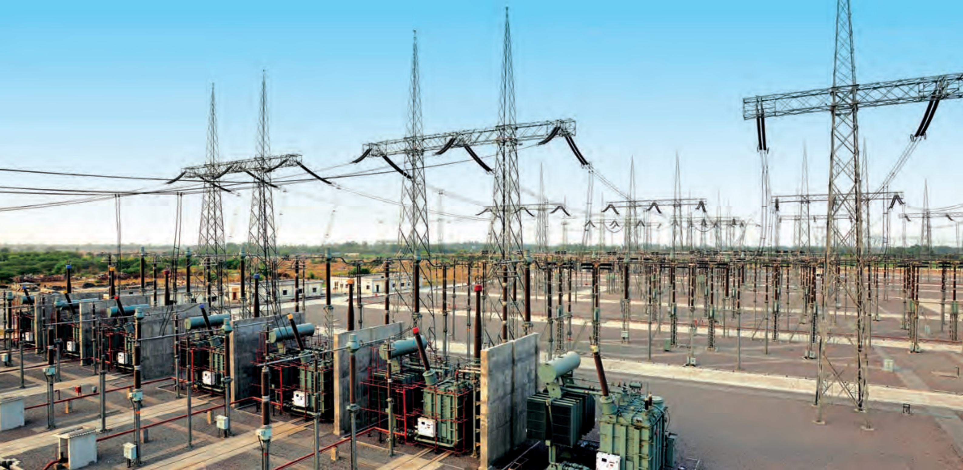
Substation incorporating 765 kV Air-Insulated Switchgear at Unnao in Uttar Pradesh. L&T offers complete solutions in high-voltage substations and power transmission lines.
