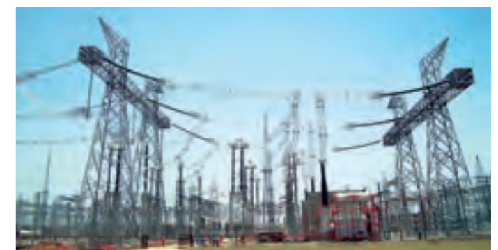
India's first 1200 kV substation at Bina in Madhya Pradesh built by L&T.
