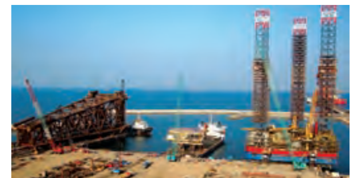
A jack-up rig along with a wellhead platform and a jacket at L&T's Modular Fabrication Yard in Sohar, Oman.
