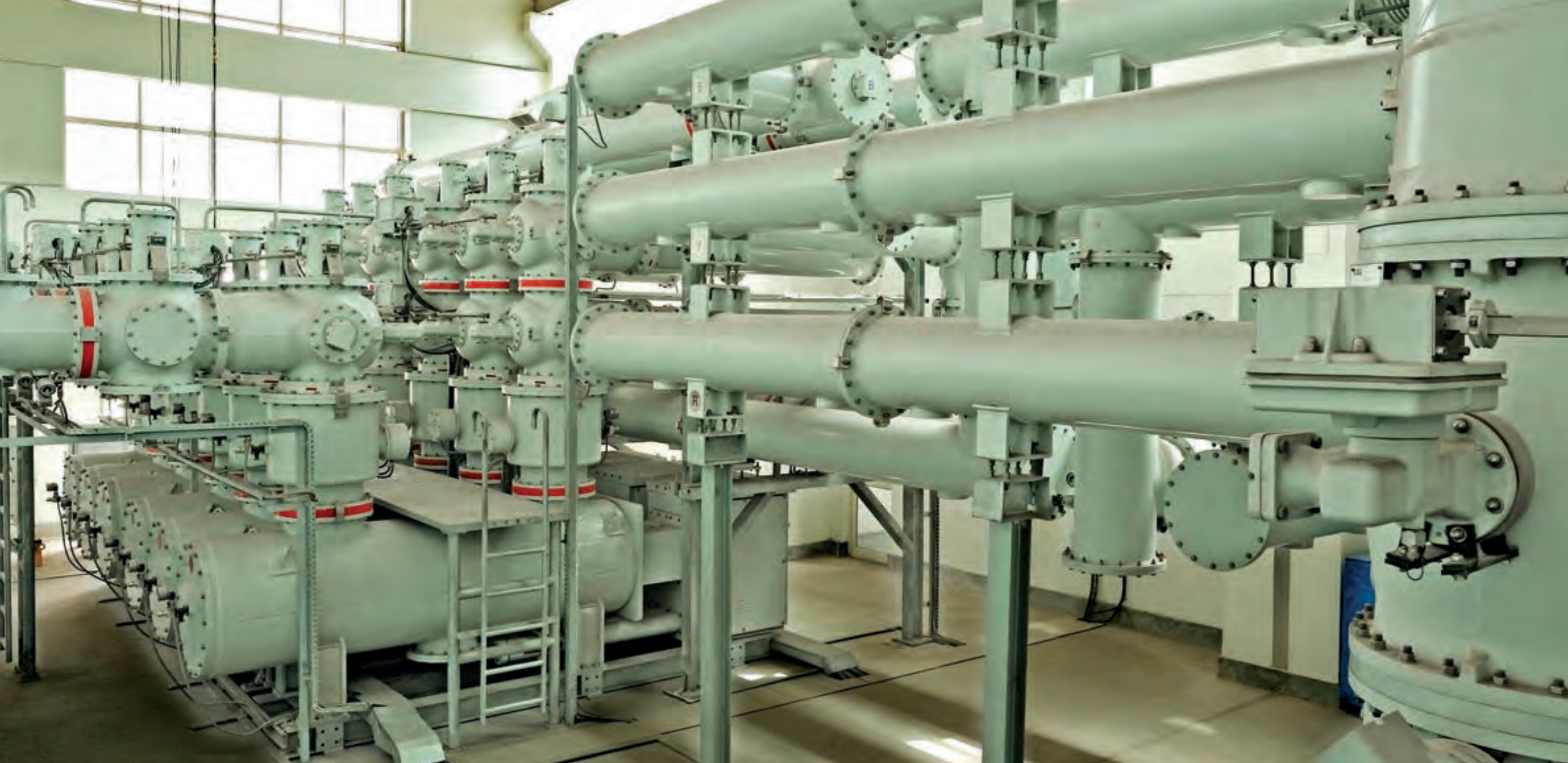
One of many 400 kV Gas-Insulated Substations (GIS) installed by L&T. The Company is one of the major players in the power transmission and distribution sector in the Middle East, with a track record extending across the UAE, Qatar, Kuwait, Oman and Saudi Arabia.
