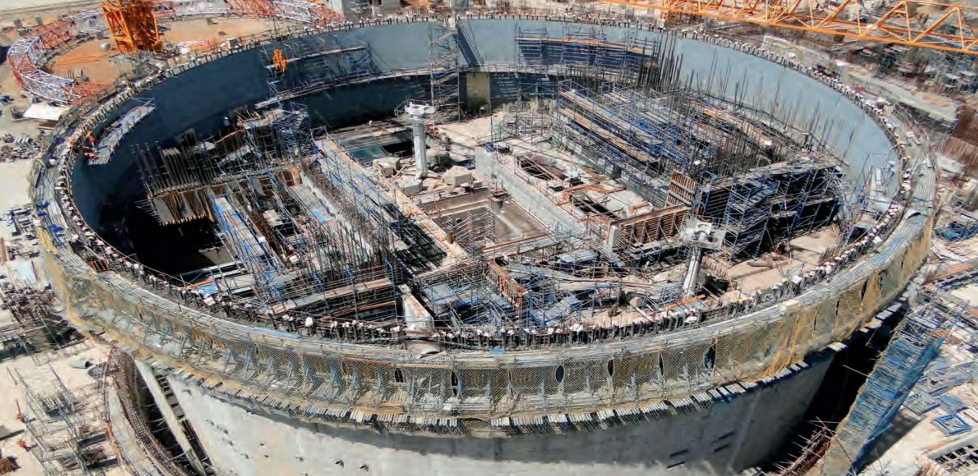
Kakrapar Atomic Power Project, Gujarat, under construction. L&T has contributed to India's nuclear power programme both through comprehensive construction of critical structures and supply of vital equipment.
