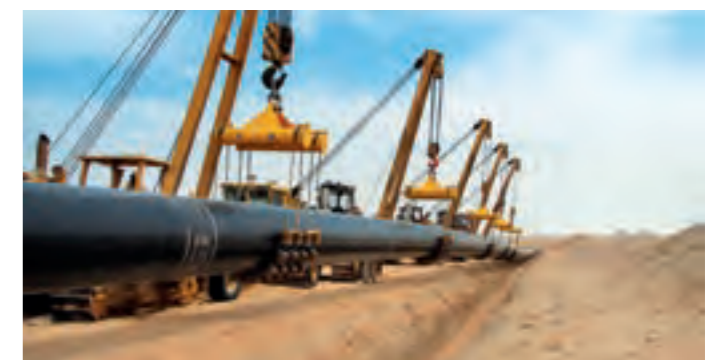
Habshan-Ruwais-Shuweihat Pipeline being executed on an EPC basis in Abu Dhabi. The track record includes over 4,000 km of pipeline across the toughest terrain.
