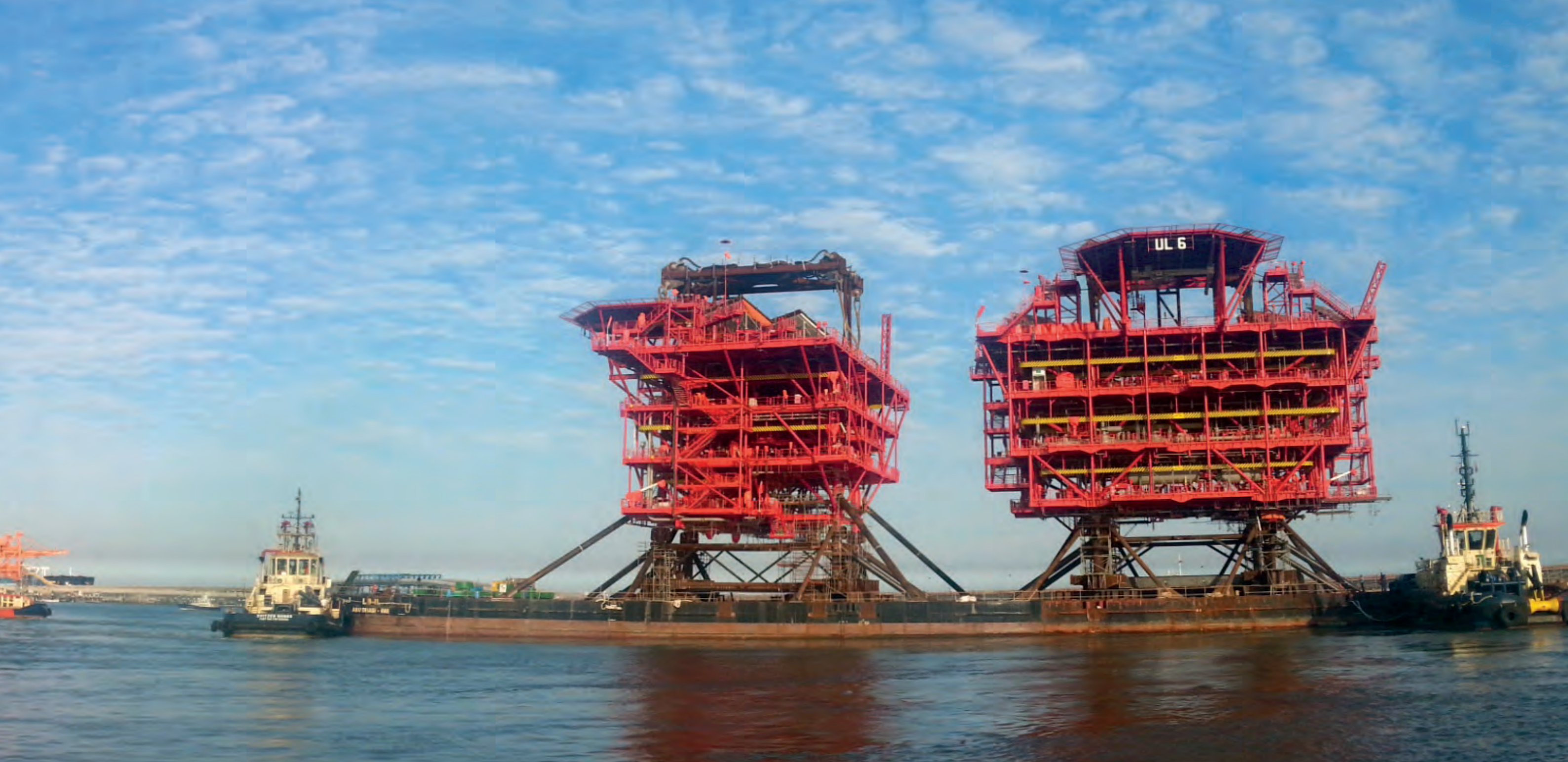
Topsides sail away from L&T Modular Fabrication Yard in Sohar, Oman for Nasr & Umm Lulu Development project of ADMA-OPCO, Abu Dhabi.
