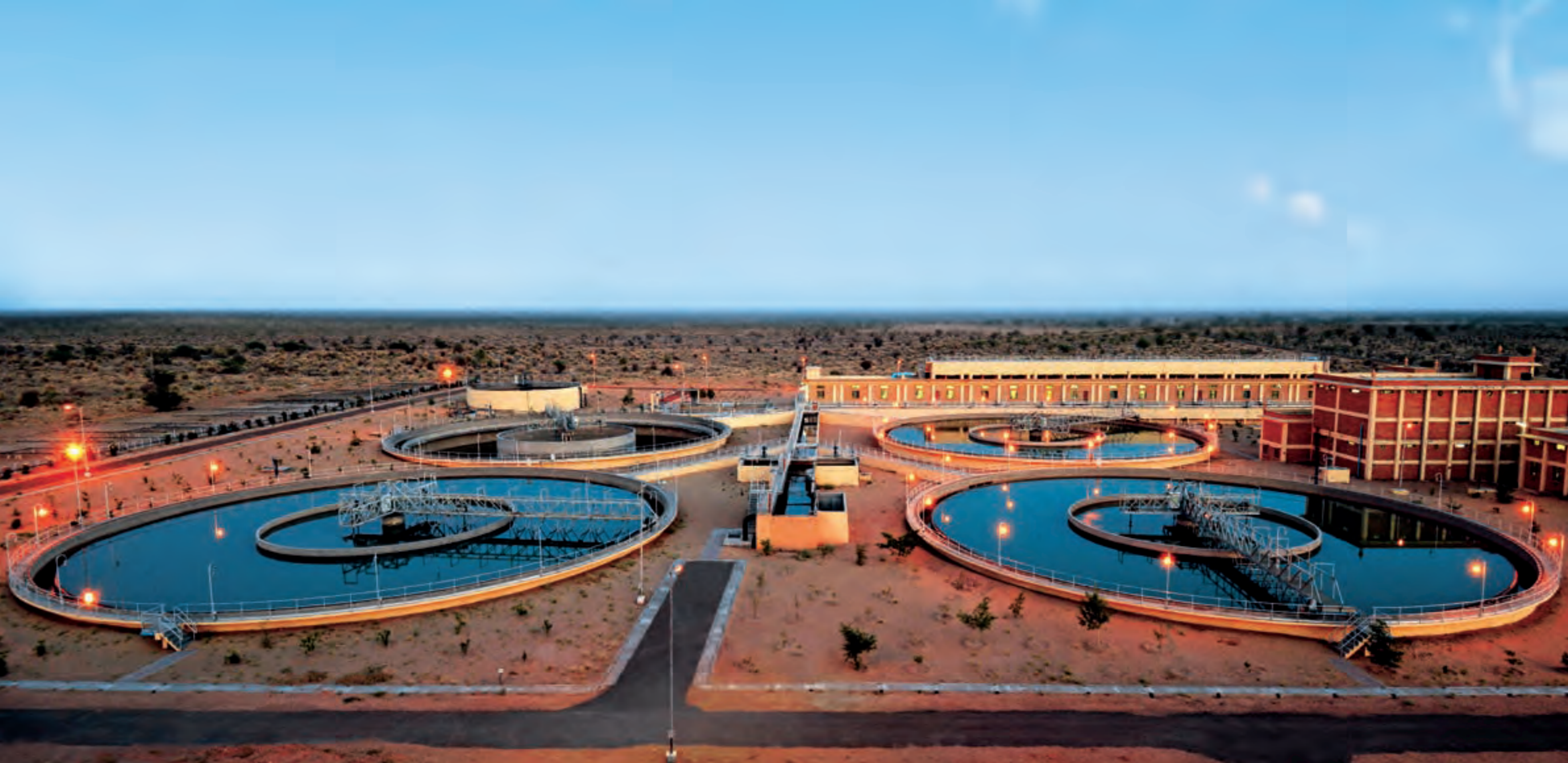
172 MLD water treatment plant for Barmer Lift Water Supply Project at Jaisalmer, Rajasthan. L&T has designed and constructed water reservoirs, pumping stations, pipeline networks and distribution systems.
