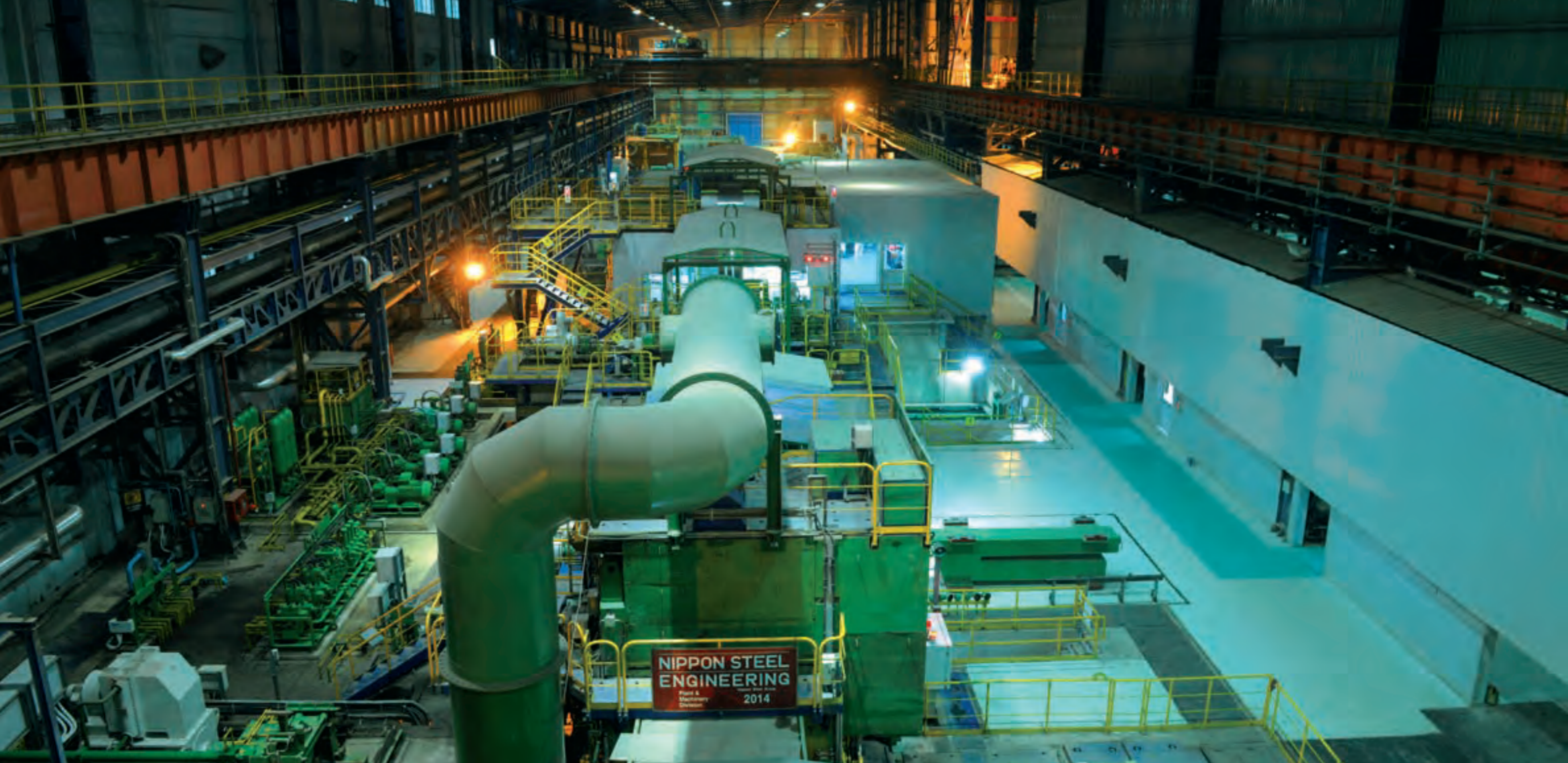
A Continuous Annealing Process Line built by L&T at Tata Steel's plant at Jamshedpur. L&T undertakes detailed engineering, procurement, manufacture, supply, construction, erection and commissioning of projects in the areas of ferrous and non-ferrous metals, and mineral beneficiation.
