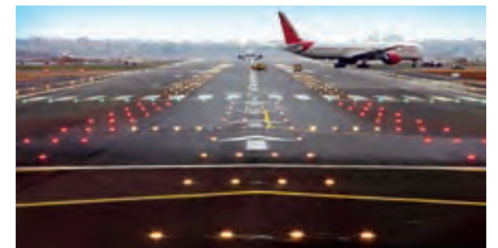
Airfield ground lighting at Mumbai International Airport. Runways built by L&T include those incorporating CAT IIIB Instrument Landing Systems.
