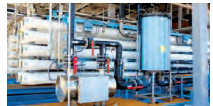
Reverse osmosis technology in operation at desalination projects.
