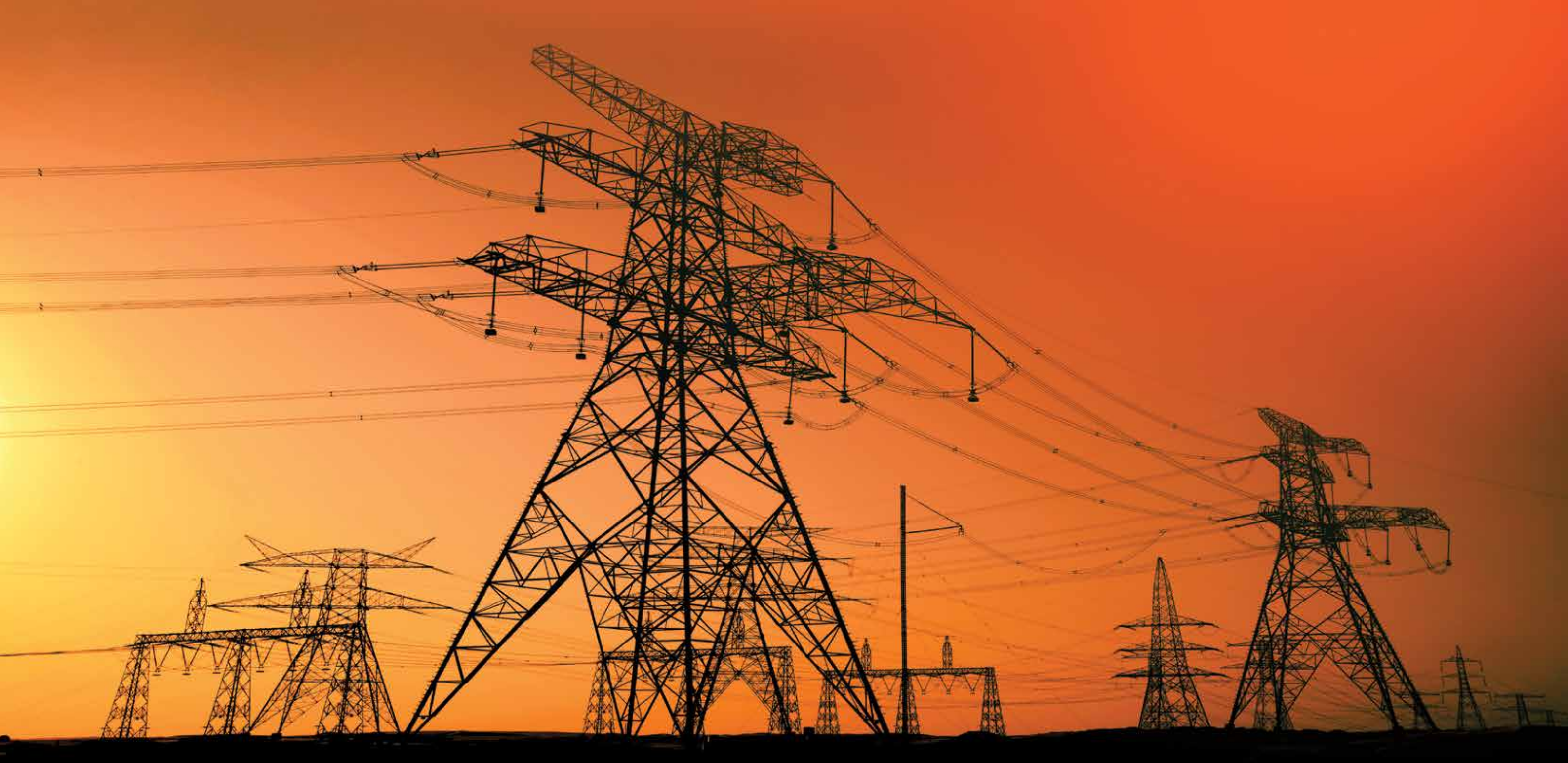
400 kV Bab Asab - Habshan Transmission Line in Abu Dhabi. L&T is one of the industry leaders in turnkey construction of power transmission and distribution systems in the Middle East.
