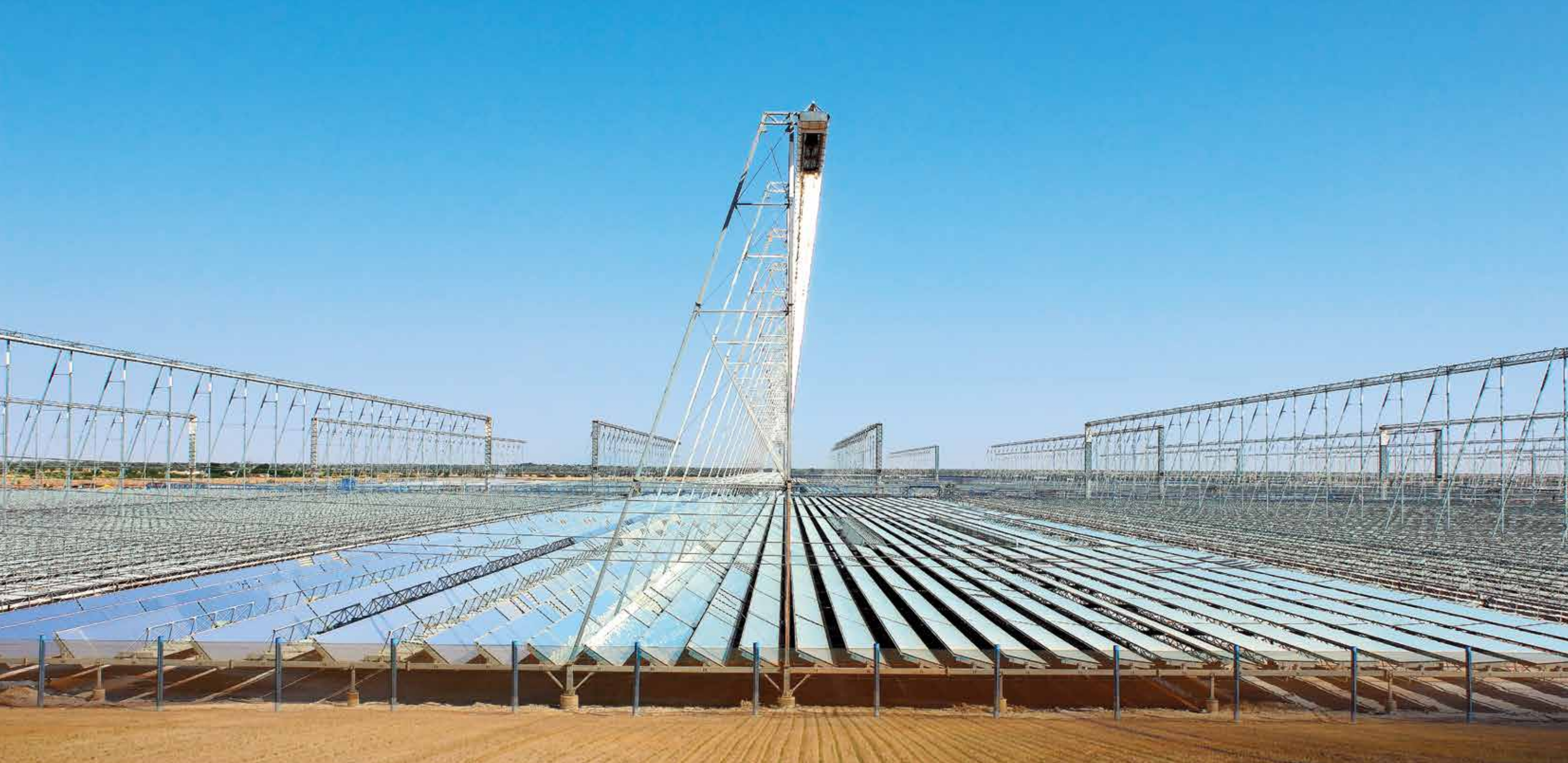
Asia's largest (125 MWe) solar thermal power plant in Rajasthan, based on high efficiency, CSP technology. L&T is the country's largest player in the field of solar plant construction.
