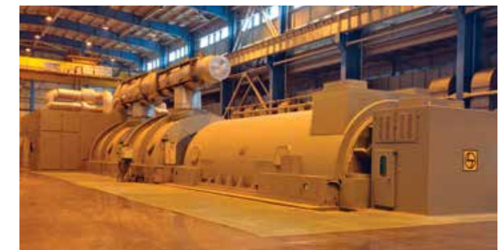
Enclosed turbine at a supercritical power project.
