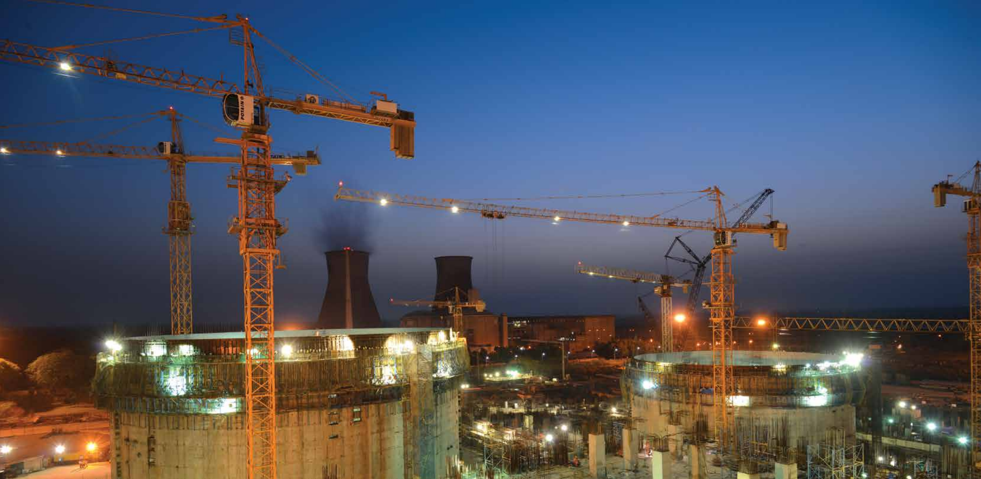
Massive construction work in progress at Kakrapar Nuclear Power Project in Gujarat. L&T has been entrusted by the Nuclear Power Corporation with critical structures for most of India's nuclear power plants.
