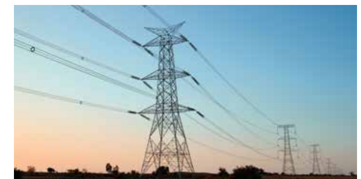
765 kV DC transmission lines at Kudgi, Karnataka.
