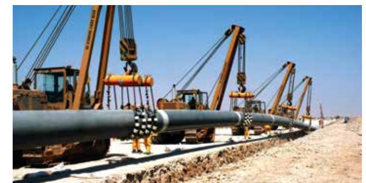
Lowering of 36" dia. gas pipeline for Qatar Petroleum at Ras Laffan. The EPC scope also included civil, mechanical, electrical and instrumentation works for three metering stations.
