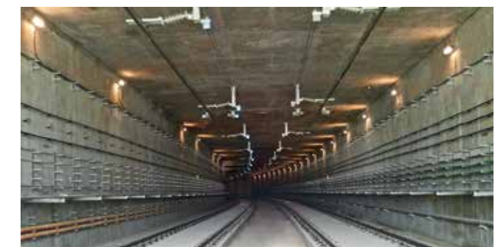
Rigid Overhead Contact System of Delhi Metro Rail Corporation.
