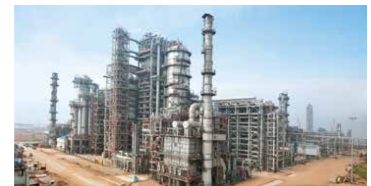
4.17 MMTPA FCCU reactor & regenerator section for IOCL's Paradip Refinery.
