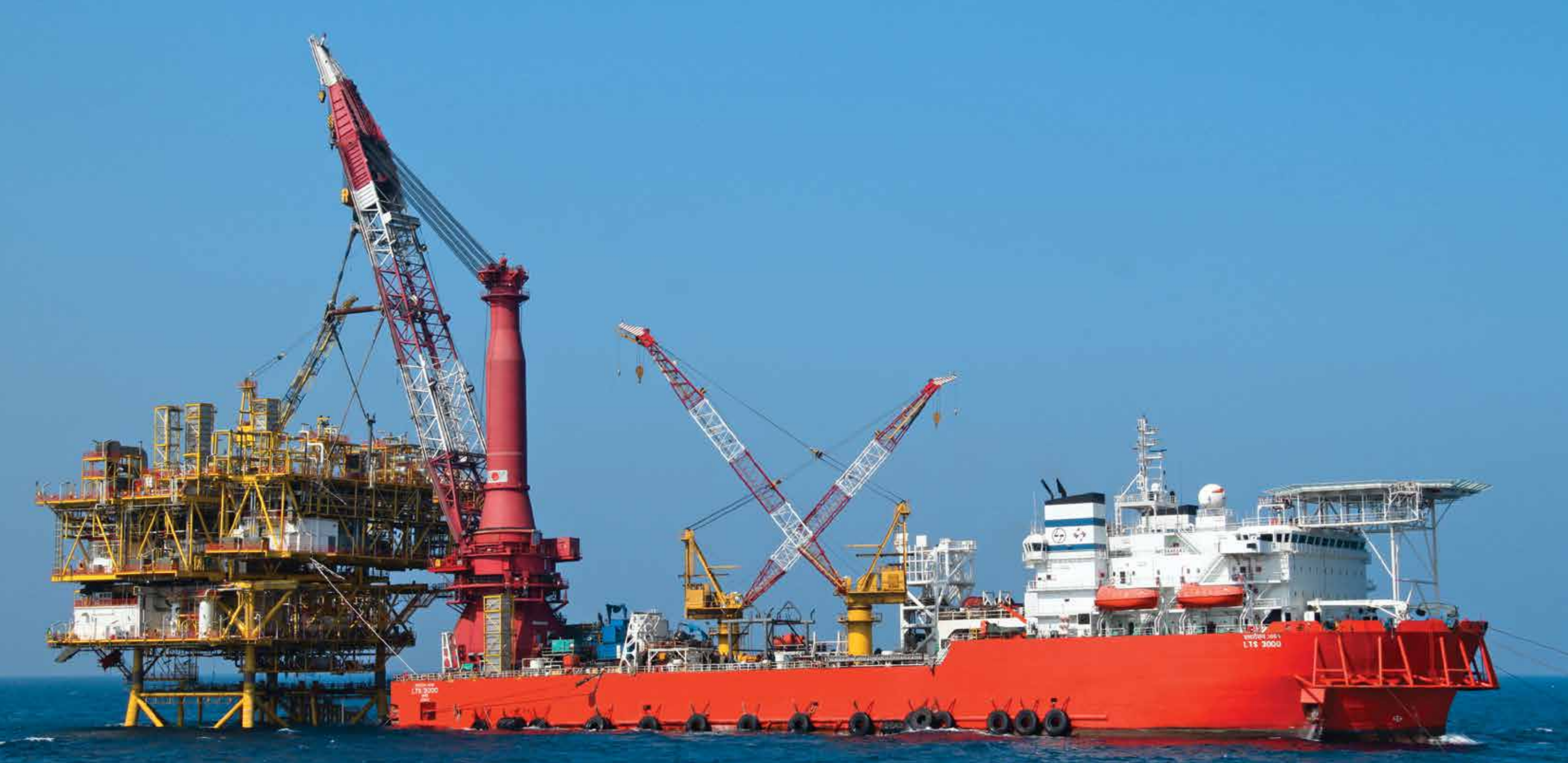
3000 tonne captive installation and pipelay vessel installs a wellhead platform at Yetagun off Myanmar. The vessel provides the Company with the installation edge for all its offshore projects.
