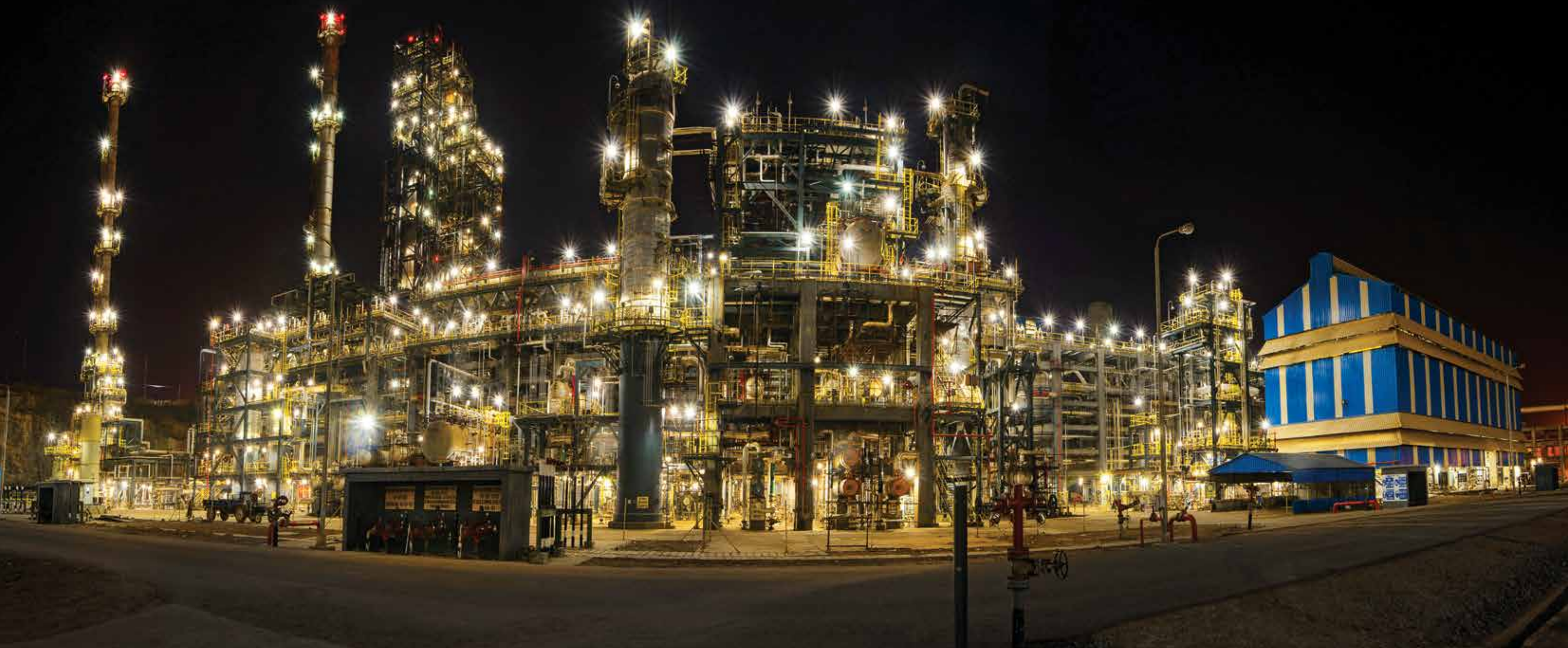
An aromatic complex built on LSTK basis for ONGC Mangalore Petrochemicals Limited in Mangalore. L&T Hydrocarbon has proven capabilities to execute critical sections of major petrochemical complexes.
