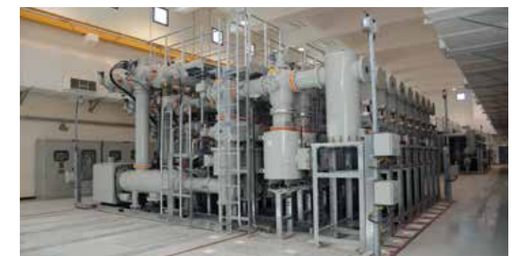
Electrical installations at the gas-based industrial super substation in Doha.
