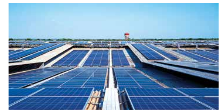
World's largest single rooftop (7.5 MWp) solar power plant in Punjab.
