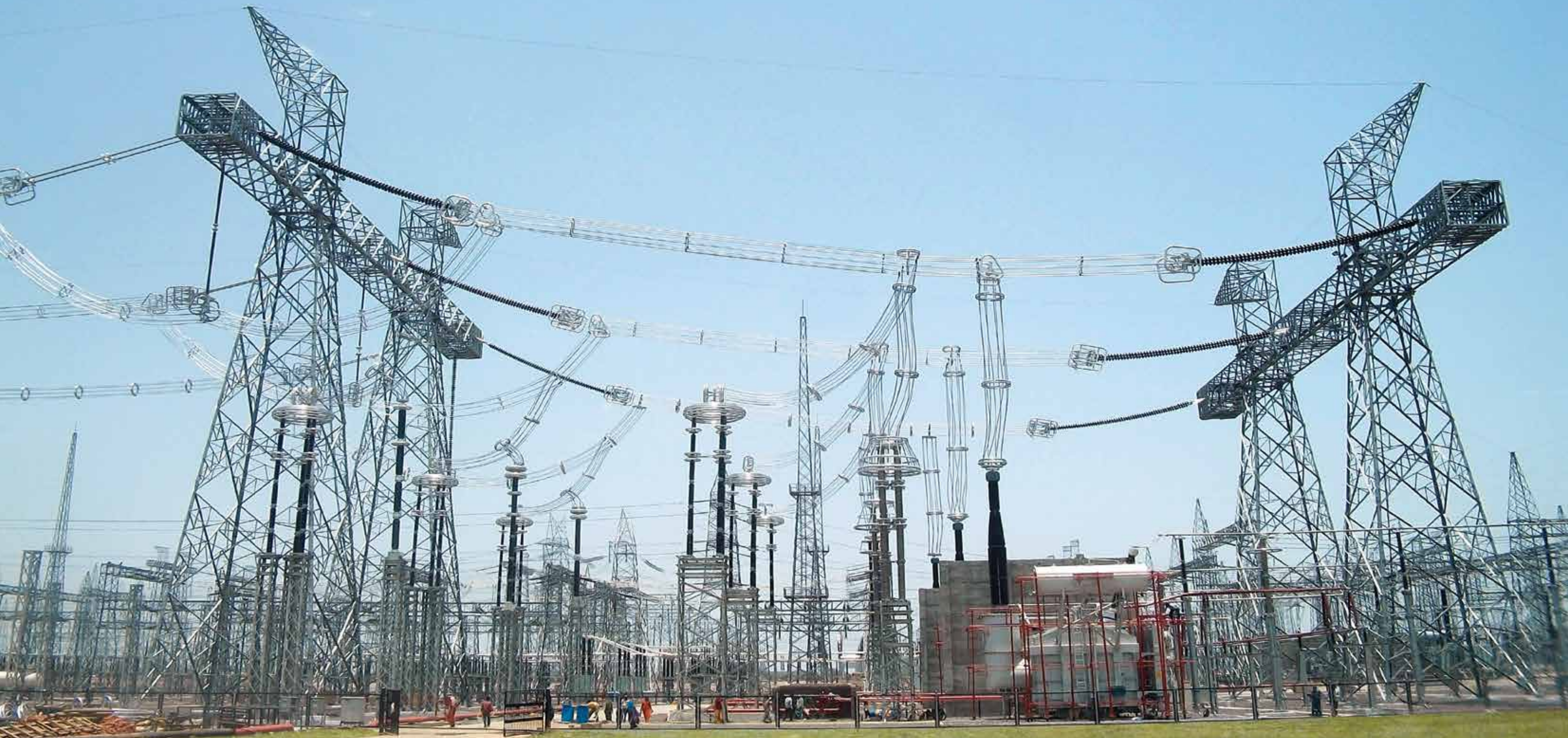
India's first 1200 kV substation at Bina in Madhya Pradesh. L&T offers complete solutions in high-voltage substations and power transmission lines.
