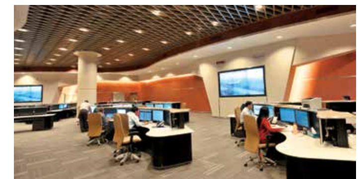
Mumbai International Airport Network Operations Centre - powered by L&T's control and automation systems and expertise.
