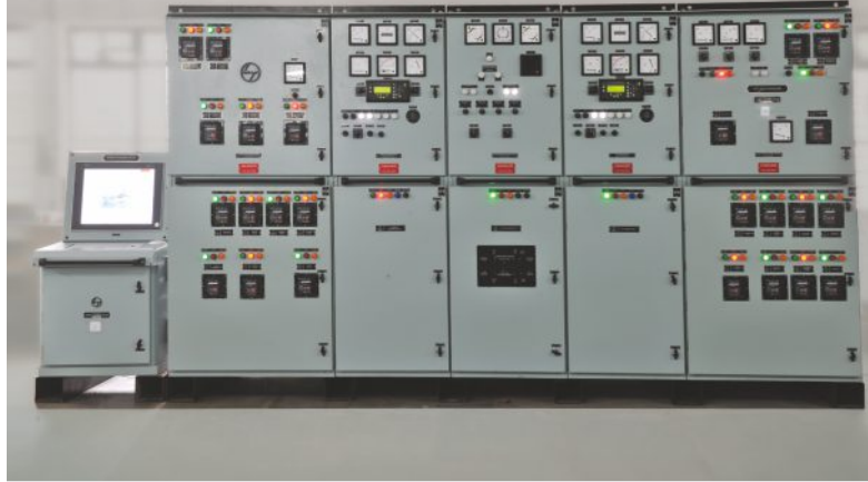
Retrofitted Main Switchboard with APMS Console
