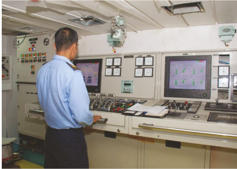
MCR Console with Platform Management System
