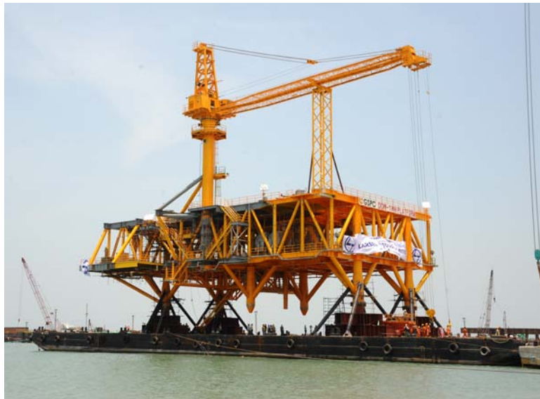
Well-head platform for GSPC poised for sail-out. Below: KV breaks a coconut on the auspicious occasion.
