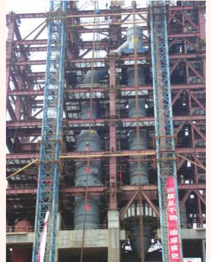
The world's largest coal gasifier manufactured by L&T being erected at a project site in China
